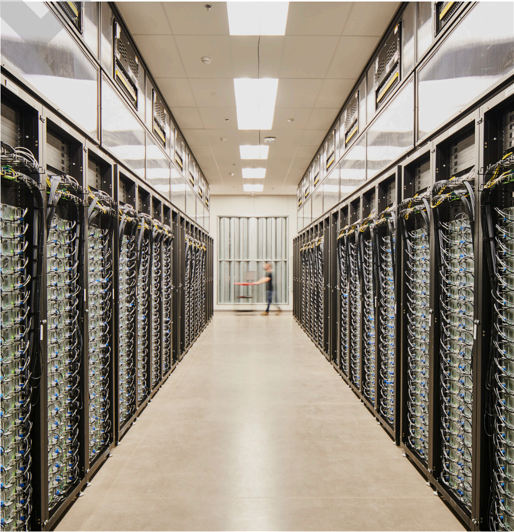
Apple's Reno data centre, which opened in 2012, takes advantage of the mild climate by cooling its servers with outside air whenever possible.
